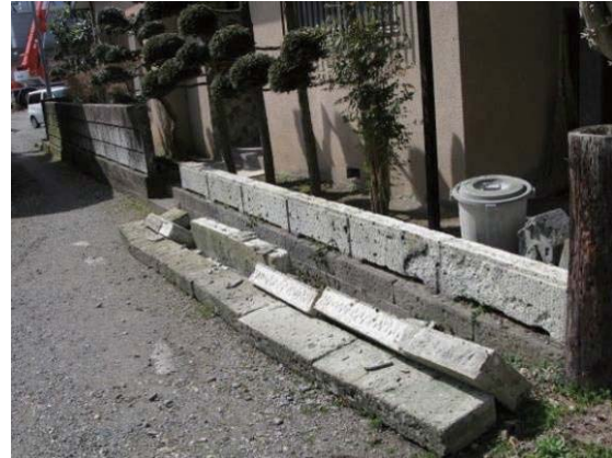
Photo 6.3-53 Collapse of stone masonry wall (Shirakawa city)
