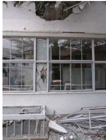
Photo 6.3-8 Shear failure of the first-story column
