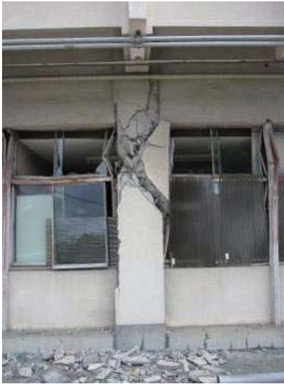
Photo 6.3-18 Shear failure of column
