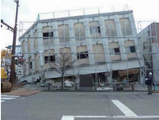
Photo 6.3-4 First-story collapsed building (Sukagawa city)
