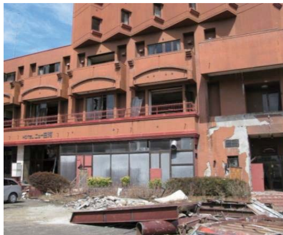
Photo 6.3-24 Appearance of damaged building (Shirakawa city, Fukushima pref.)
