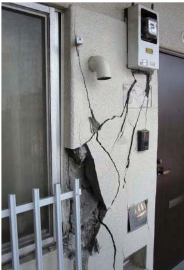
Photo 6.3-30 Shear cracks on nonstructural wall
