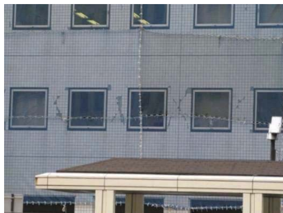
Photo 6.3-49 Damage of tile on exterior wall
