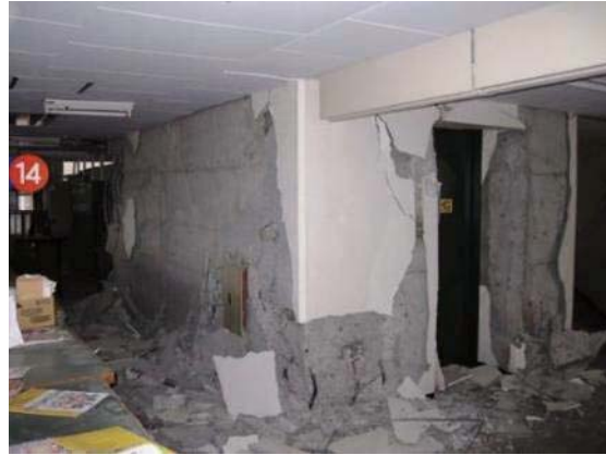
Photo 6.3-16 Failure of shear wall
