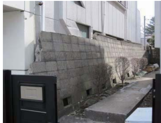
Photo 6.3-51 Collapse of concrete block wall (Sukagawa city)
