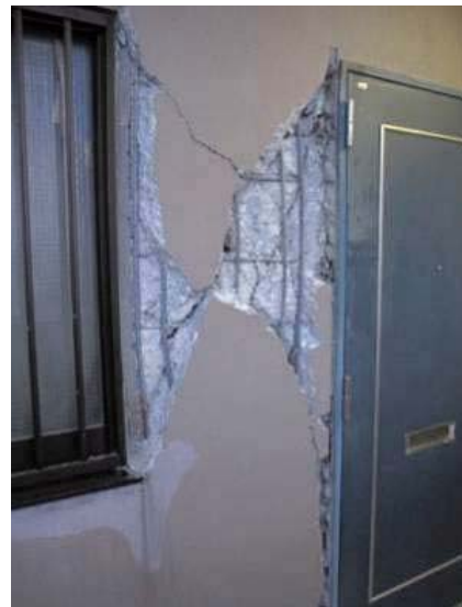
Photo 6.3-42 Shear failure of nonstructural wall
