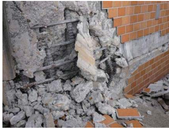
Photo 6.3-23 Damage at the bottom of SRC column
