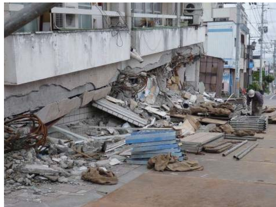
Photo 6.3-3 Close-up view of the fallen first story
