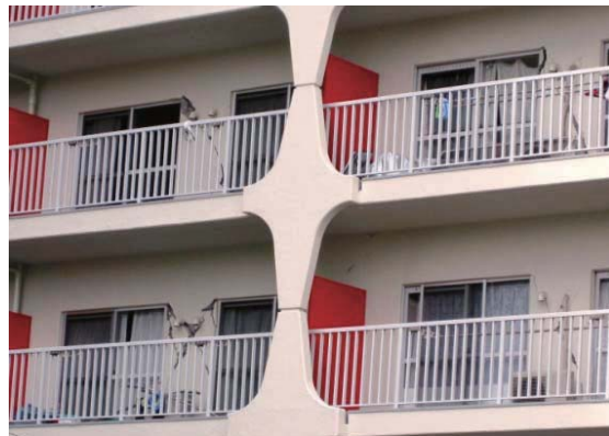
Photo 6.3-31 Shear cracks on mullion
