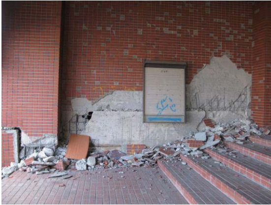
Photo 6.3-25 Damage of the bottom of SRC column and shear wall
