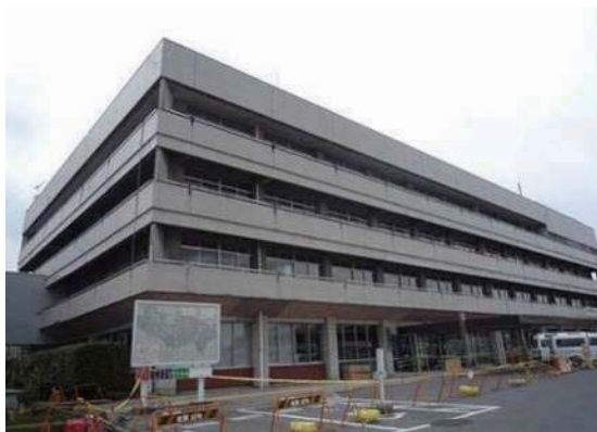
Photo 6.3-14 Appearance of damaged building (Sukagawa city)
