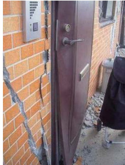
Photo 6.3-44 Damage of nonstructural wall and deformed door in same building shown in Photo 6.3-22
