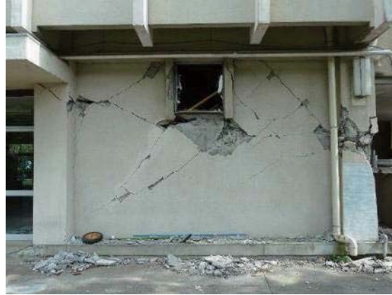
Photo 6.3-19 Shear failure of wall with opening
