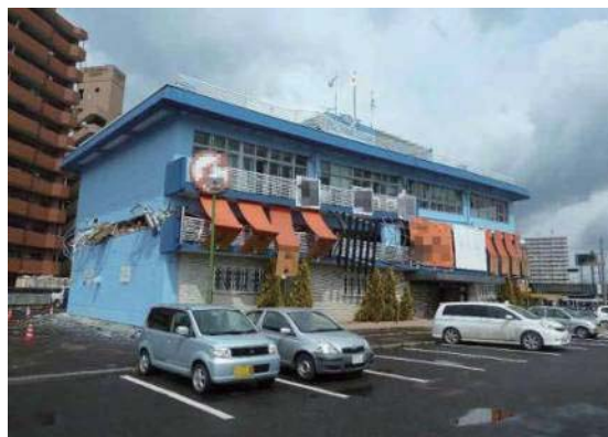
Photo 6.3-6 Mid-story collapsed building (Wakabayashi ward, Sendai city)
