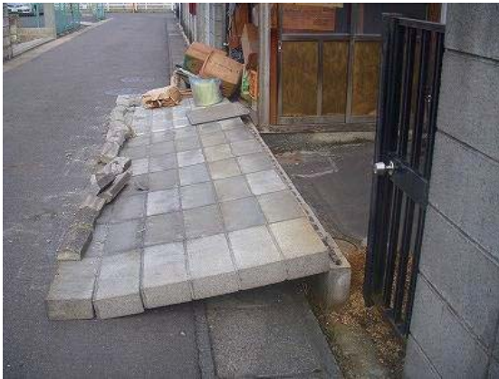
Photo 6.3-50 Collapse of concrete block wall (Koriyama city)
