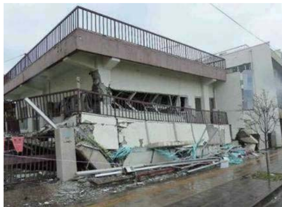
Photo 6.3-1 First-story collapsed building (Wakabayashi ward, Sendai city)
