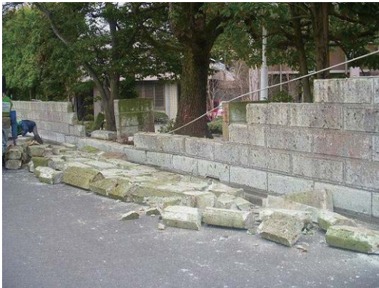
Photo 6.3-52 Collapse of stone masonry wall (Fukushima city)
