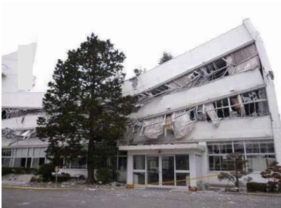
Photo 6.3-7 Mid-story collapsed building (Fukushima city)
