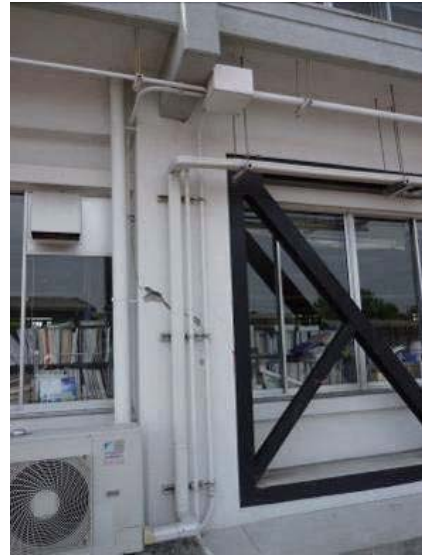
Photo 6.3-38 Shear crack on column with framed steel braces
