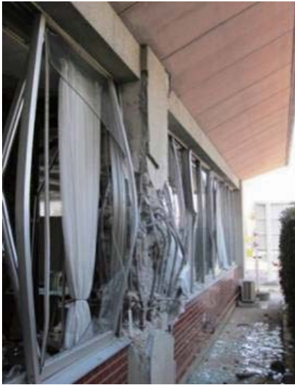
Photo 6.3-15 Shear failure of short column
