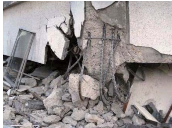
Photo 6.3-5 Close-up view of the fallen story
