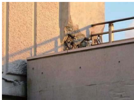
Photo 6.3-21 Crushing at the bottom of column of the multi-story shear wall
