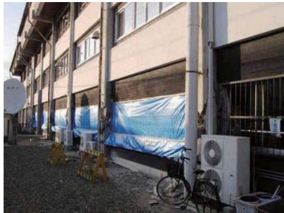
Photo 6.3-9 Appearance of the damaged building (Tono city)
