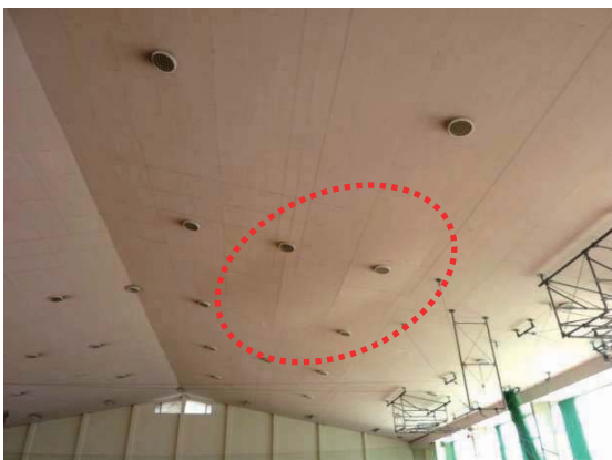
Photo 6.6-19 Sagging of metal furring suspended ceiling
