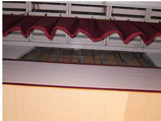
Photo 6.6-23 Falling of cement mortar finish above stage
