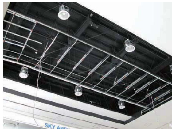
Photo 6.6-16 Falling of metal furring suspended ceiling
