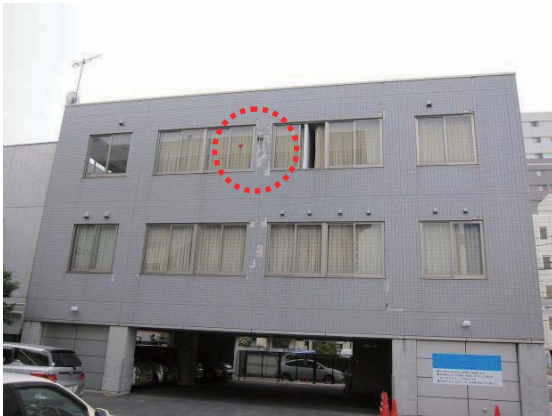
Photo 6.6-6 Falling of ceramic wall tiles and breakage of AAC panels
