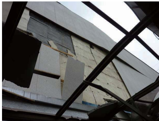
Photo 6.6-5 Damage to gymnasium gable end wall
