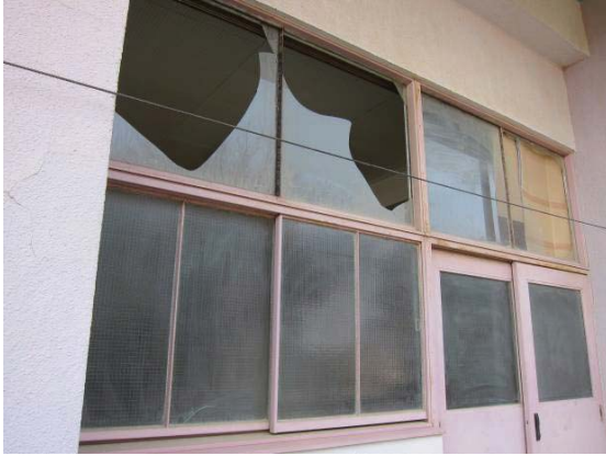
Photo 6.6-9 Breakage of window glasses installed to fixed window frame with hardening putty
