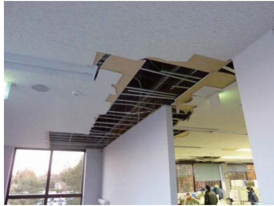
Photo 6.6-22 Damage to metal furring suspended ceiling at the connection
