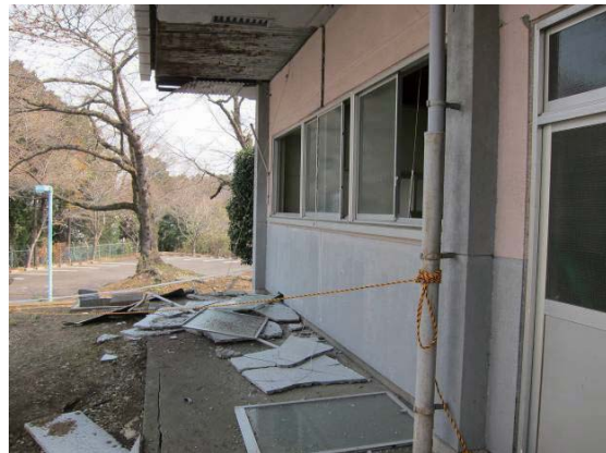
Photo 6.6-4 Falling of cement mortar and metal lath from eaves soffit
