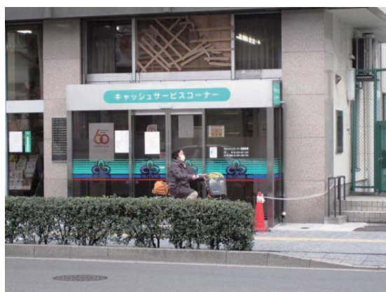
Photo 6.6-8 Broken window glass
