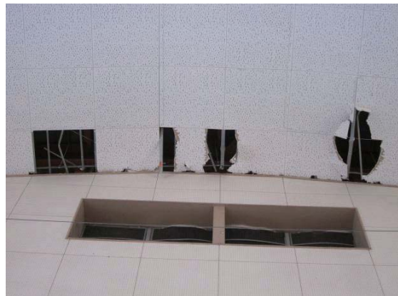
Photo 6.6-20 Damage to metal furring ceiling at the connection wall
