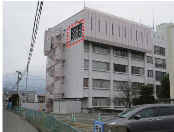
Photo 6.6-7 Detachment of AAC panels
