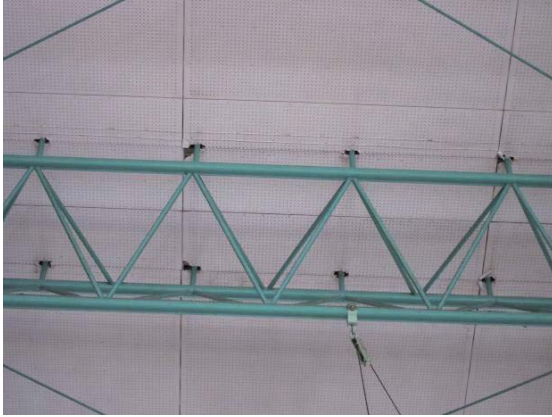
Photo 6.6-21 Damage to metal furring suspended ceiling at the connection
