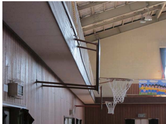
Photo 6.6-25 Damaged interior wall
