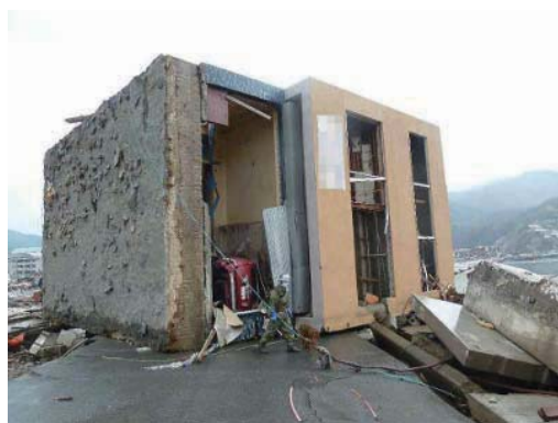
Photo 7.2-2 Overturning of a 3-story reinforced concrete building
