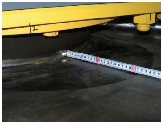
Photo 9.2-24 Trace of displacement of elastic sliding bearing
