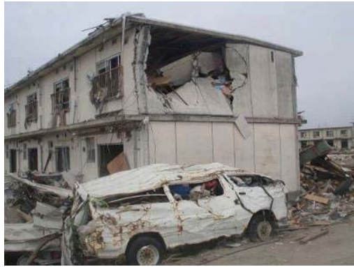
Photo 7.2-6 Wall opening probably generated by debris impact
