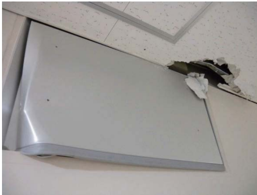
(a) Damage to the panel
