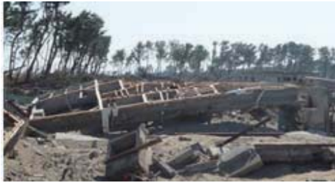
Photo.7.4-1. Foundations washed away.
