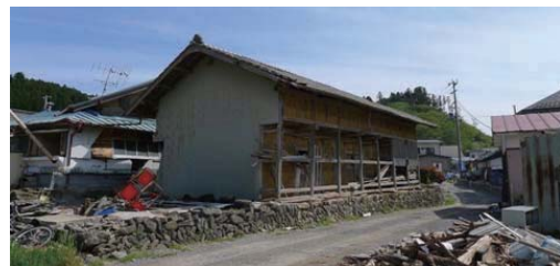
Photo 7.4-32. Survived soil warehouse (10) which seemed to have comparatively slight structural specifications in Akasaki-cho, Oofunato city.
