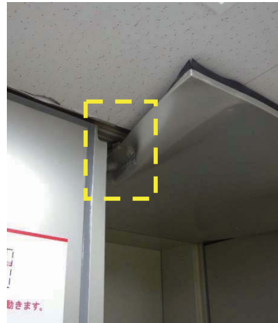
(b) Damage to the expansion joint
