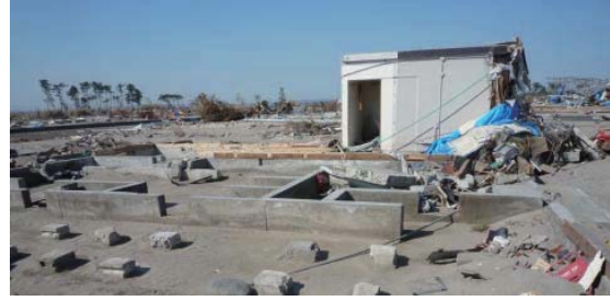
Photo.7.4-2. Only foundation remained.
