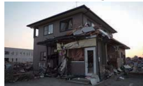
Photo 7.4-13. Wood house with store ( 5 ) remained in the downstream of the survived buildings in Yuriage.
