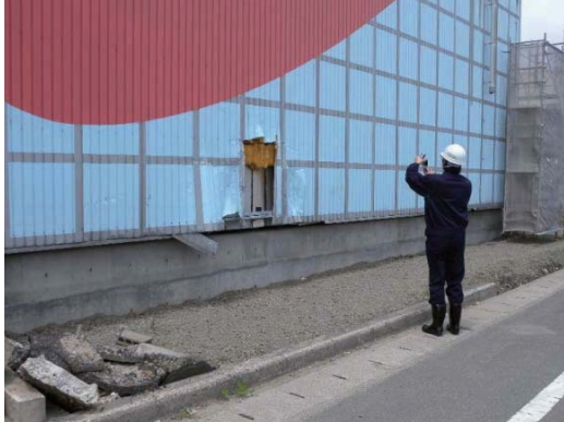
Photo 9.2-6 Damage due to debris
