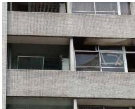
Photo 8.3-4 Fire scene at a condominium (Sendai city, Miyagi prefecture)
