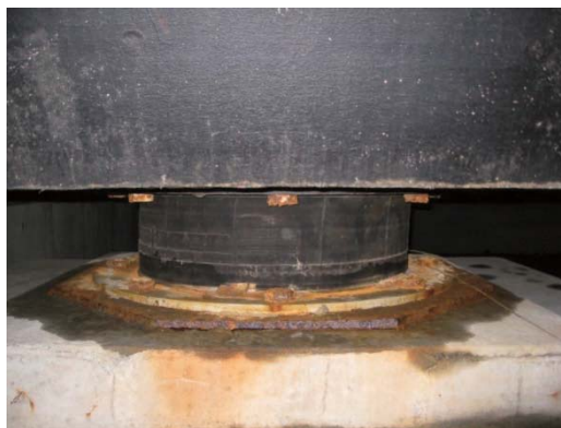
Photo 9.2-10 Rust of High-damping rubber bearing
