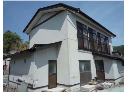
Photo 7.4-28. Wood house (3) without damage under the water depth of over 7 m in Akasaki-cho, Oofunato city.
