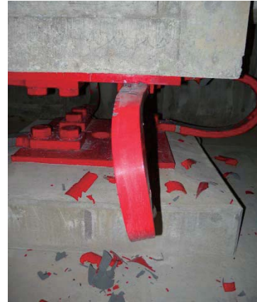
(2) Deformation of steel
