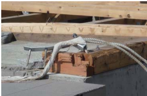
Photo.7.4-5. Failed hold down fastener.
