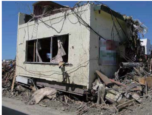
Photo 7.2-1 Story collapse of a 2-story reinforced concreted building
