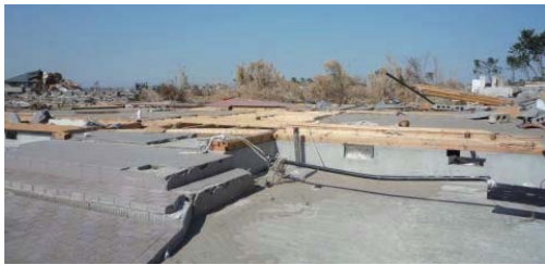
Photo.7.4-3. Foundation and sills remained.
