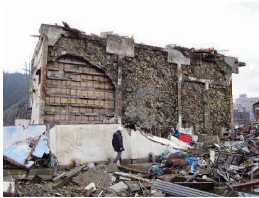
Photo 7.2-3 A 2-story reinforced concrete building that moved over the fence and overturned
