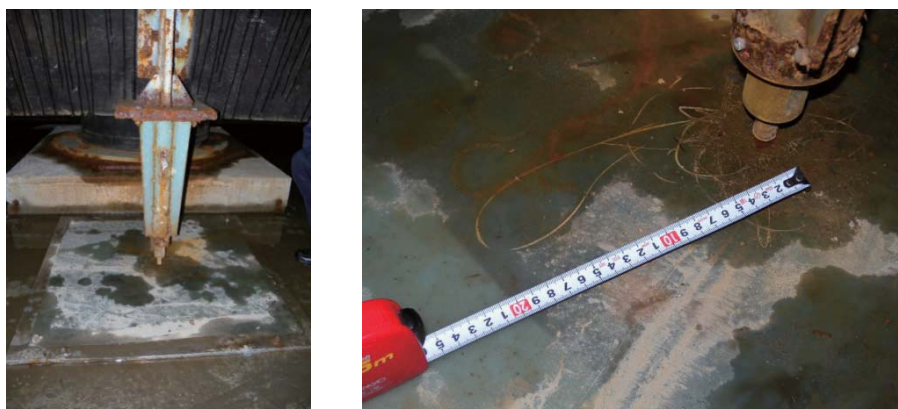
Photo 9.2-11 Trace of displacement of the SI floor on the scratch board
