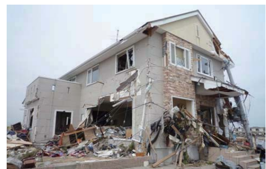
Photo 7.4-19. Light frame construction wood house (12) remained alone
