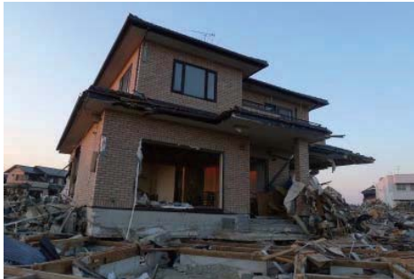
Photo 7.4-10. Wood house ( 1 ) that was carried away with the base in Yuriage, Natori city.
