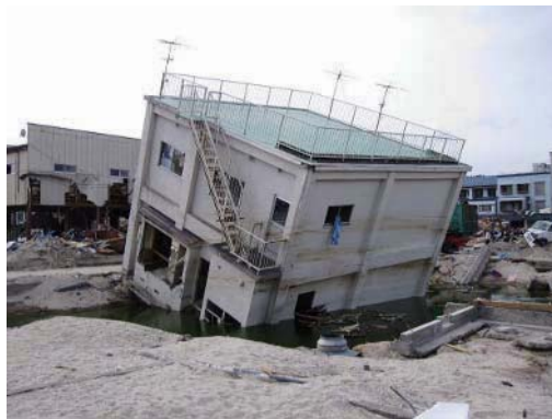
Photo 7.2-4 A 2-story reinforced concrete building that was tilted by scouring
