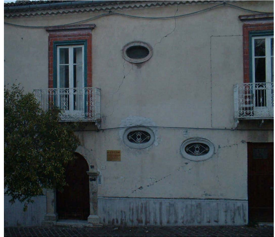
Diagonal oriented cracks up to the upper portion of solid wall - Damage grade II
