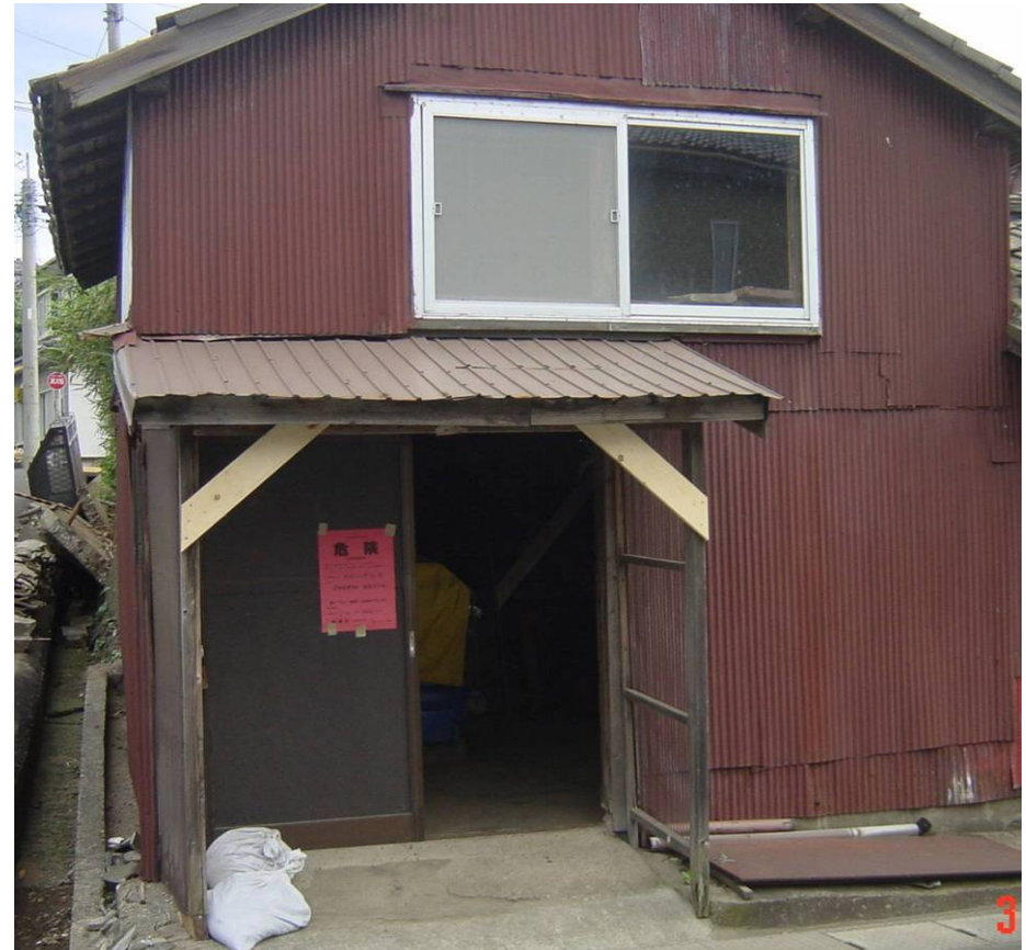
Red placard posted after Nigaata earthquake (16, July 2007)
