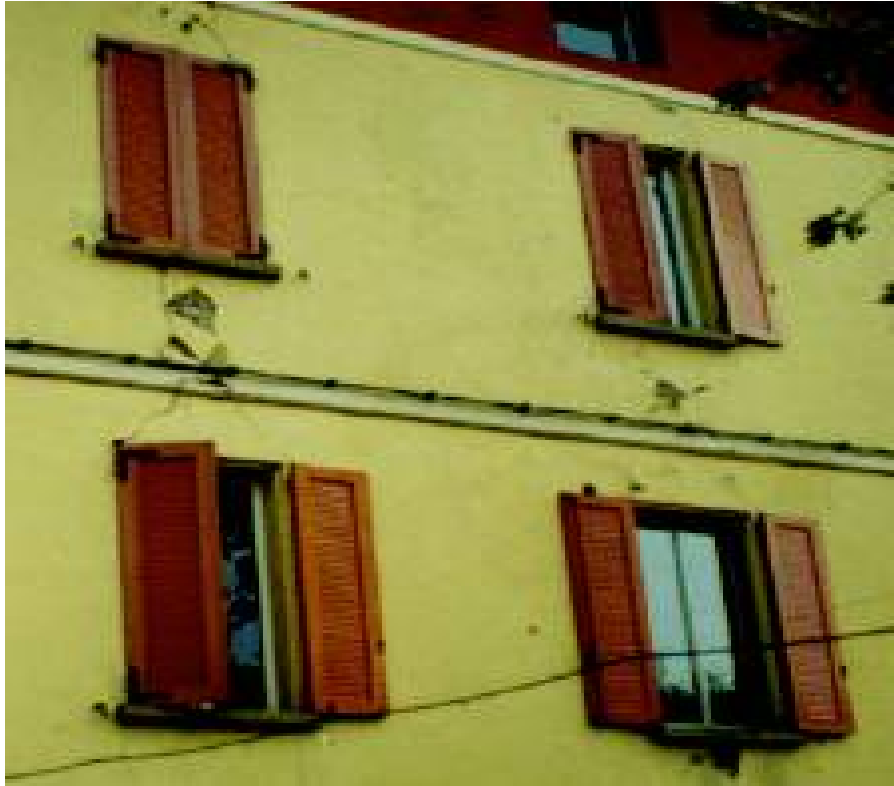
Hairlines cracks in the splendor portion of wall - Damage grade I
